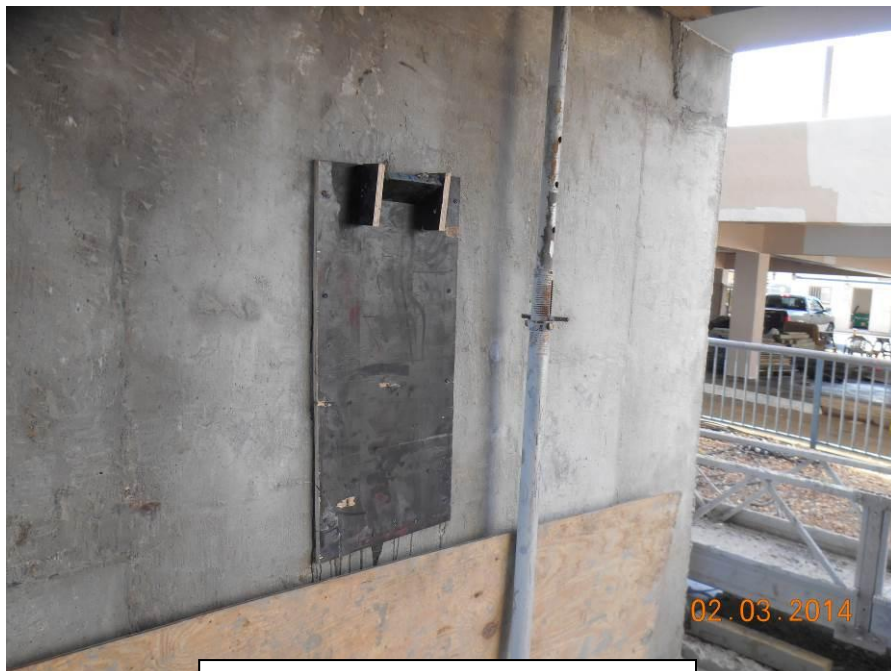
Concrete spall excavated with form built on east parking garage shearwall.
