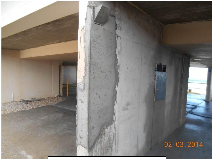
East parking garage concrete spall cast back with form removed.
